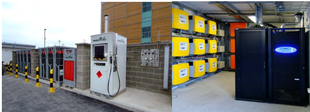
Hydrogen Storage & Dispenser
