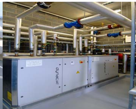
Ground Source Heat Pumps
